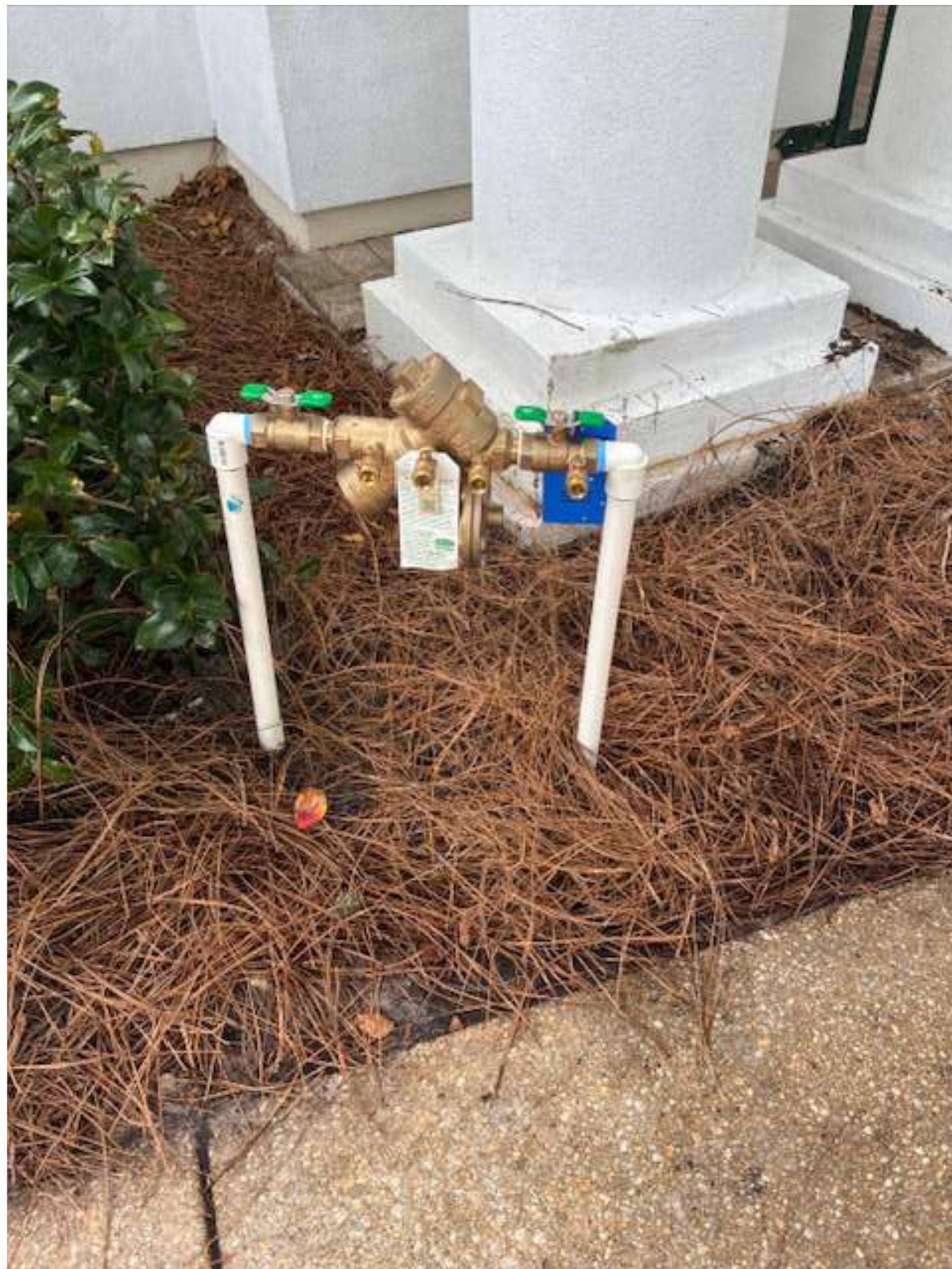
Back Flow Preventer Installed
