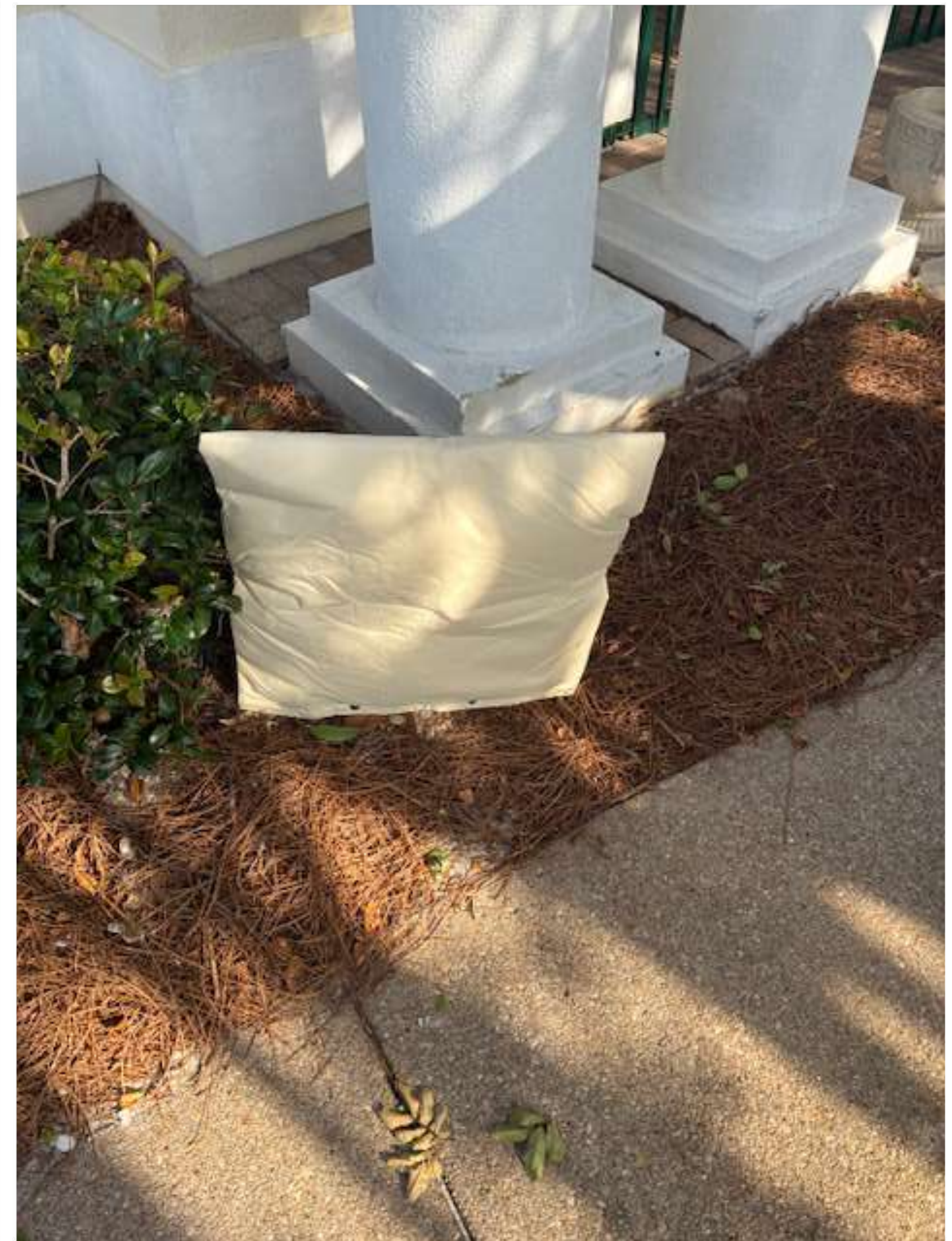
Back Flow Insulator Installed
