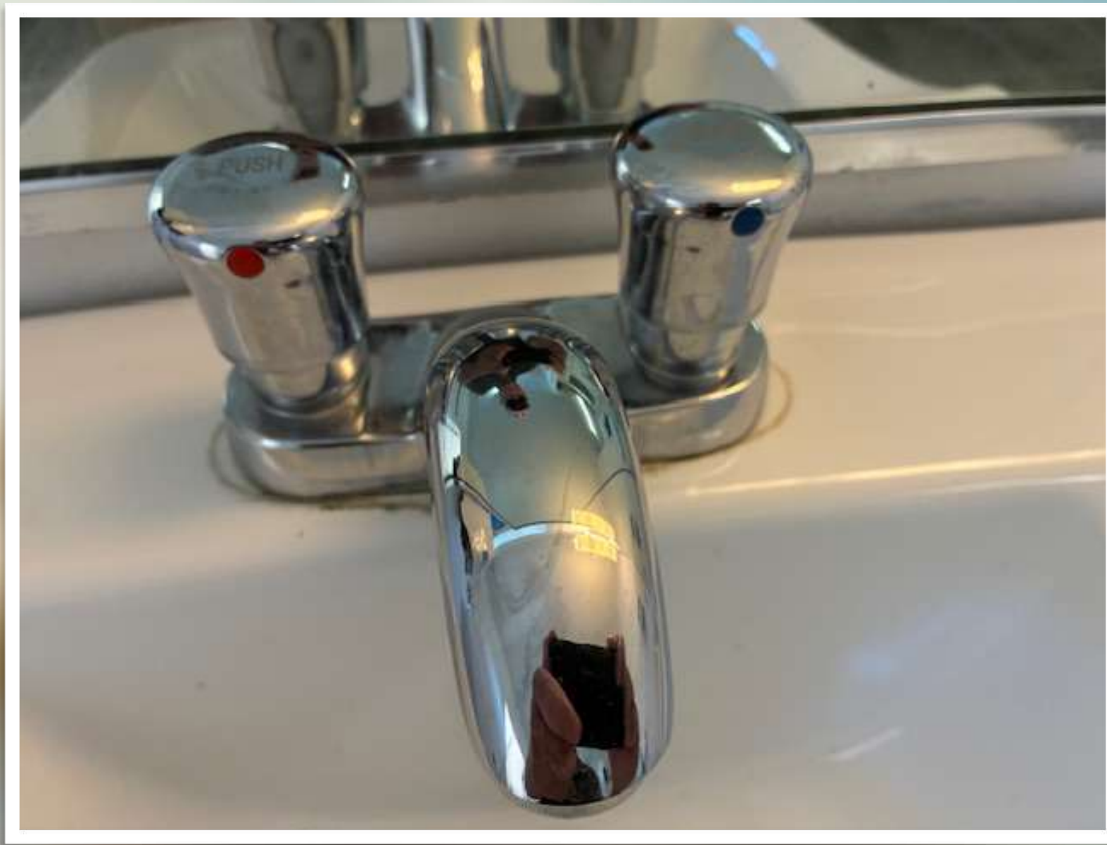
New Shut Off Faucets
